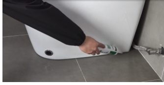
15. Apply some glass glue to fix the toilet and insulate the outside dirt from entering. (The glass adhesive in the picture needs to be purchased by oneself.)
